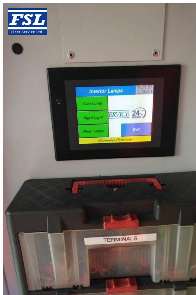
Workshop Control Interior Lights
