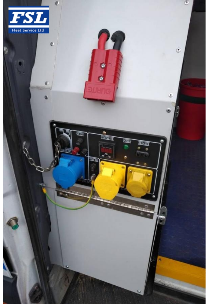
Generator Start Panel
